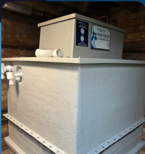
New water storage tank
